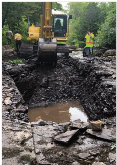
Part of the work in the Bass Lake Creek project involved digging a hole that was later covered by a thick layer of spawning gravel.
