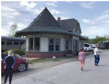
The iconic "witch's hat" of the Uxbridge Railway Station, moments after a tornado went through Uxbridge and blew out most of the station's antique windows.
