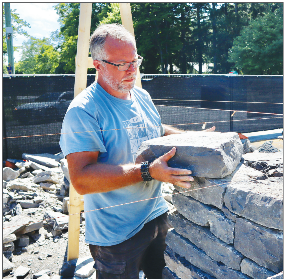
Menno Braam lays a cut stone carefully onto the east corner of the gateway wall.
