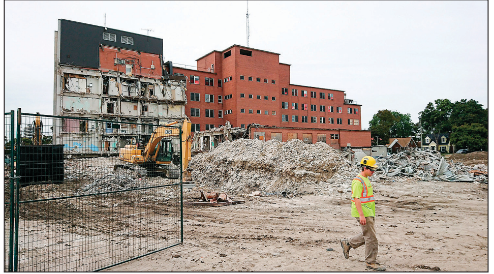
COPPER THIEVES HAVE made a small fortune off the former Sarnia General Hospital since it closed in 2011.
